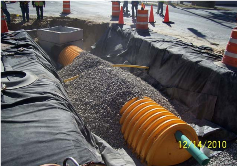
StormTech Chambers with filter fabric wrap and stone
