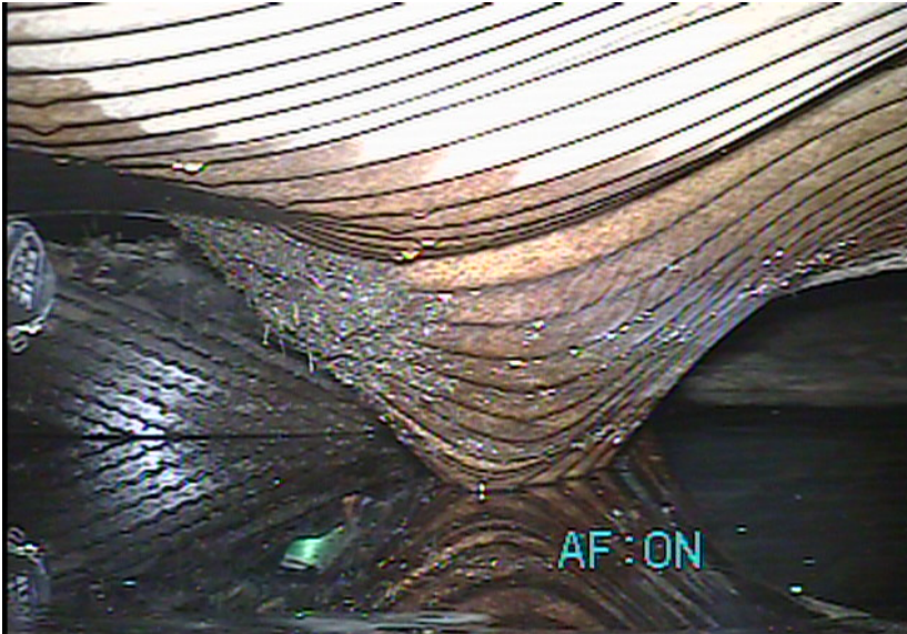
View inside crushed pipe between Pine Avenue and Jackson Street
