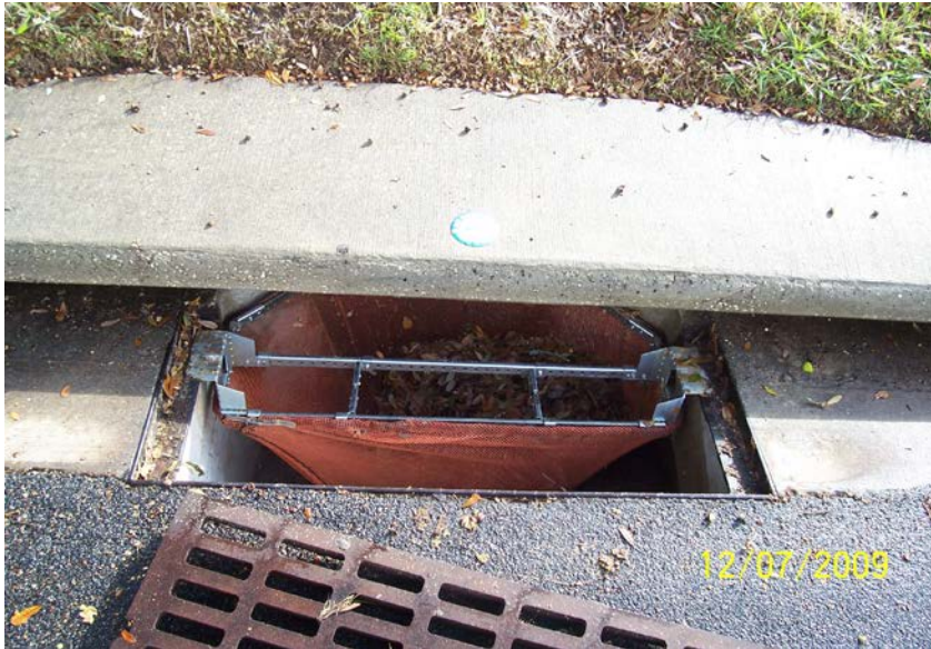
Flexstorm inlet filter at 6th Avenue and McDonald Street
